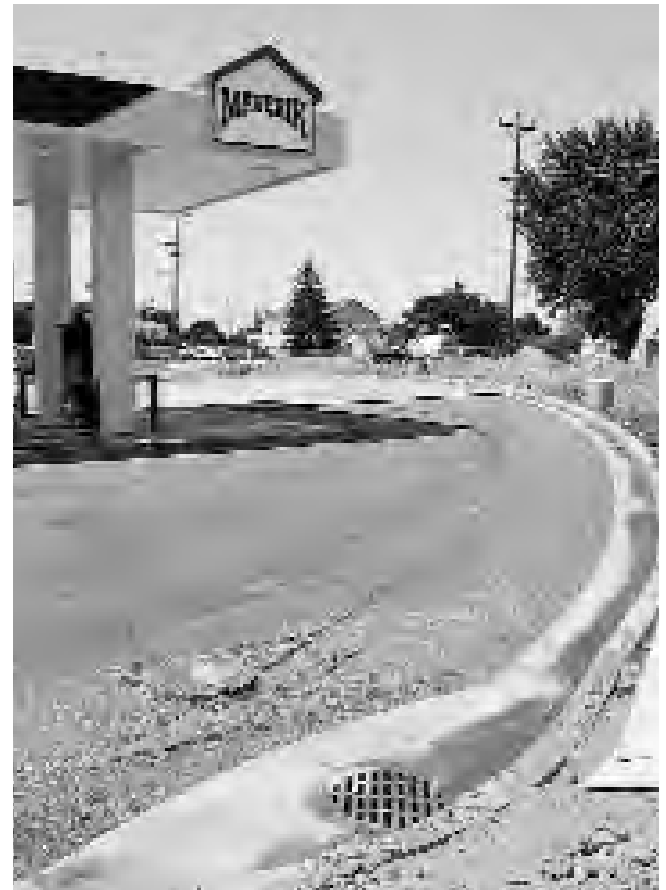
Above: Nearly completed installation of a stormwater detention system at a gas station in Nampa, ID. This site has three separate Rainstore 3 chambers to provide the necessary water storage. This photo shows the catch basin and curbing for one of the chambers. Asphalt will cover the visible gravel base.
