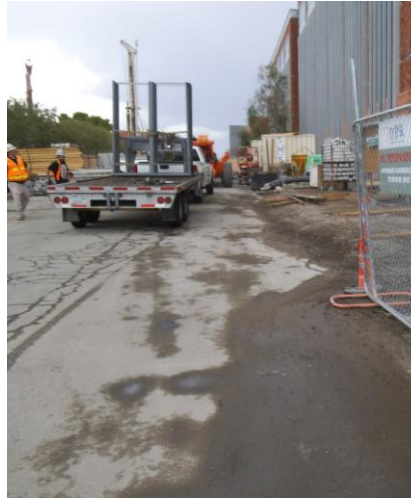
Uncontrolled sediment discharge to streets
