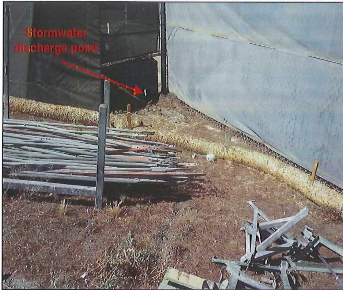
Photograph 11. View of straw wattle BMPs installed immediately upgradient of a stormwater discharge point in the southwest corner of the staging area. The straw wattles were staked down; however, they were not entrenched in the ground.
