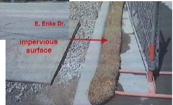
Improper BMP installation
